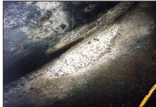
Cavitation damage is evident after proper surface cleaning
